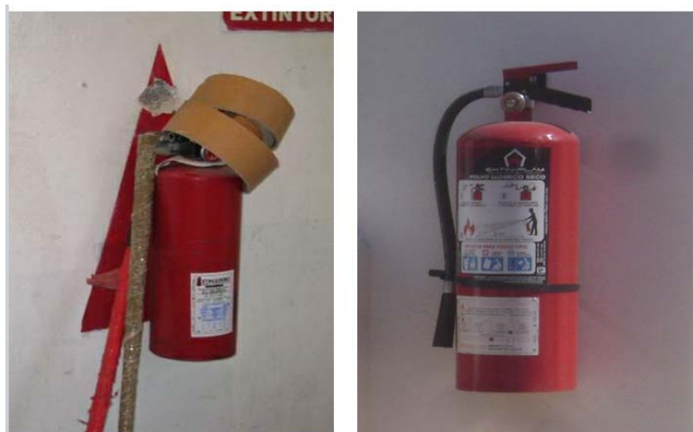
Figure 5. Corrective action in fire extinguishers
