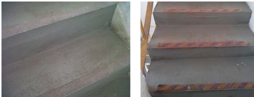
Figure 2. Non-skid tape in stairs
